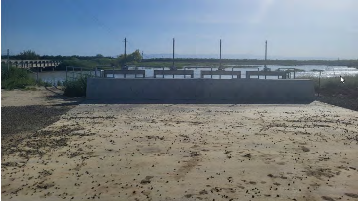
Four turnout gates on the Kings River diverting water into the Terranova Ranch canal system.
